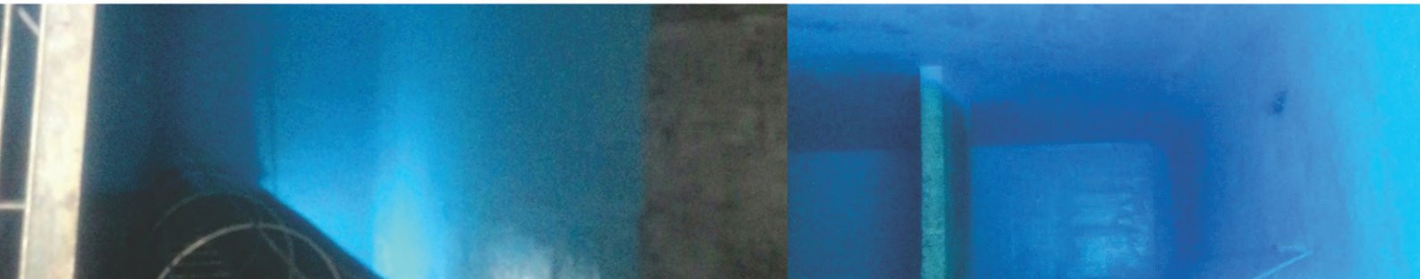
Menara Astra Ground Water Tank (GWT)
